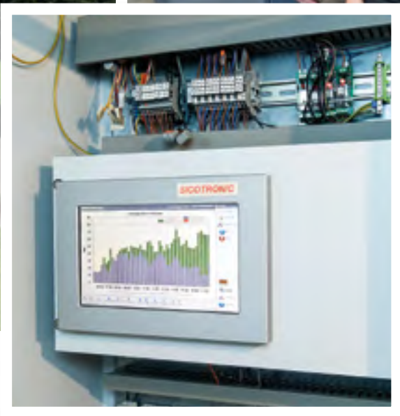
The new energy optimisation plant is the heart of the new system. It combines and monitors all electrical appliances with a connection power of more than one kilowatt.
