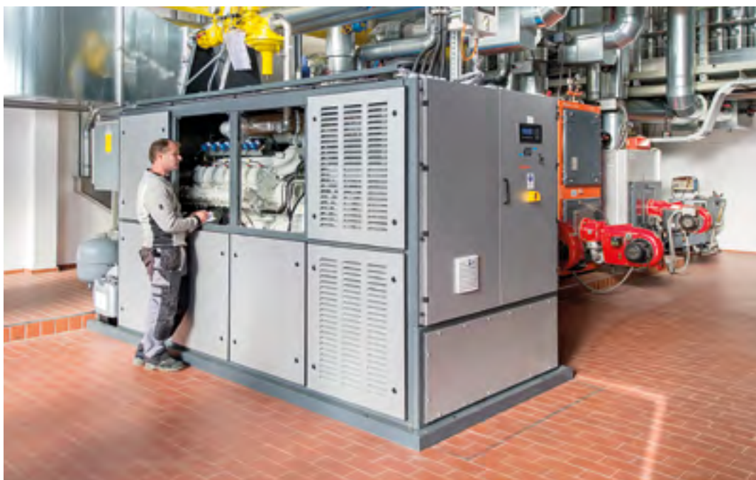
The new unit-type heating power station in Bünde is leading to an improved energy and environmental balance.
